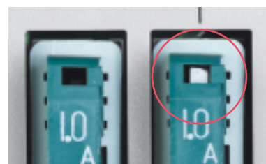
Fuse blowout indication
